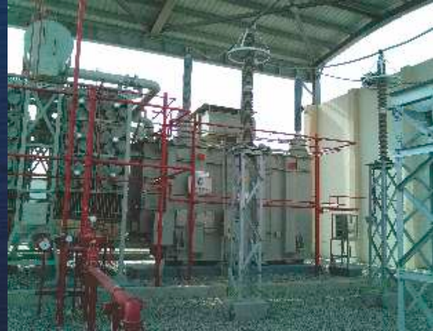
125 MVA Power Transformer at OETC 132 kV Rusail Grid Station, Sultanate of Oman
